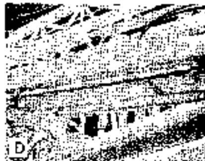
D Retainer pins installed to secure both ends of front gantry support rods to jib
