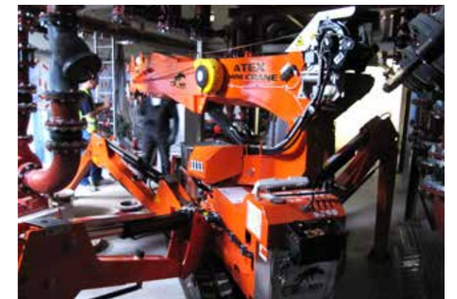
SPD360, working inside an oil plant
