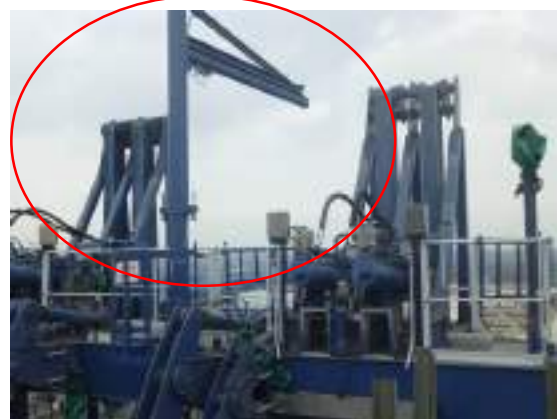
Figure 1-42: Jib Crane on Girder End
