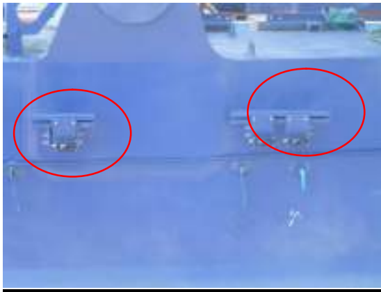
Figure 1-22 Magnetic Inductive Limit Switches nearby Boom Heel end.
