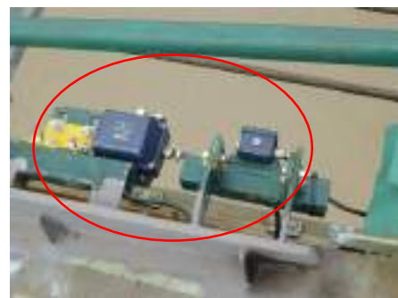
Figure 1-21:Roller Lever Operated and Magnetic Inductive Limit Switches around Boom Forward End.
