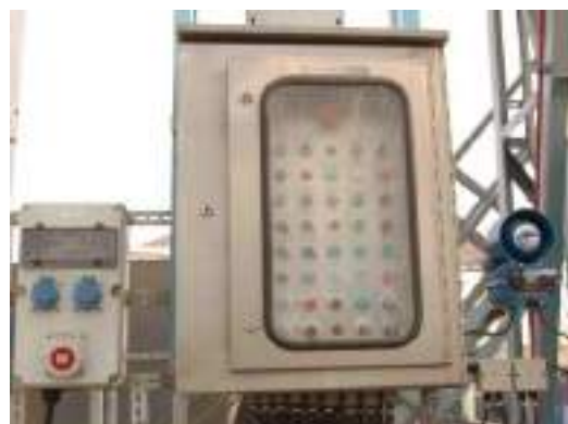
Figure 1-33: Gantry Maintenance Cab
