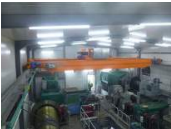
Figure 1-40: Service Crane in Machinery House
