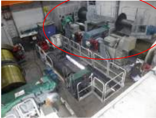
Figure 1-43: Re-reeving Device Mounted Over the Main Hoist Drive
