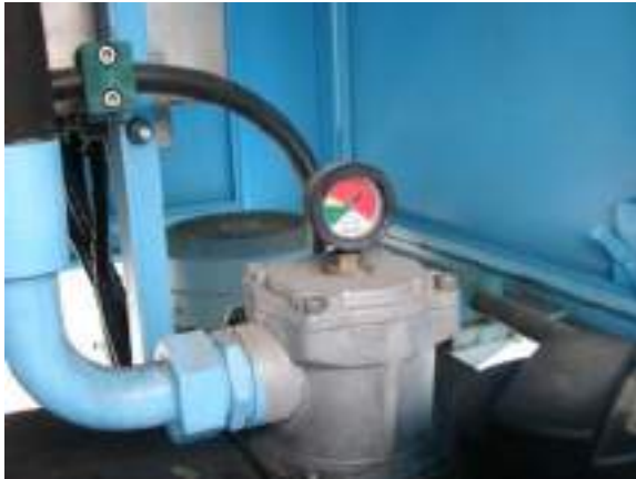
Figure 2-7: Filter of the hydraulic power package located on the girder
