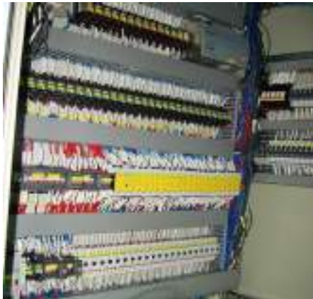
Figure 2-5: PLC controlling panel
